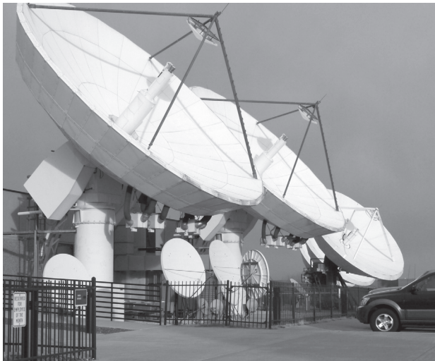
Figure I.9. A few of the several dozen transmitting antennas at EchoStar's Network's uplink facility in Cheyenne, Wyoming.
